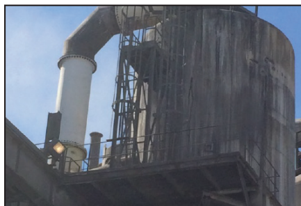
Flash cooler with exhausters.
