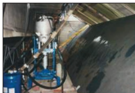
Pitting repaired using ARC 858 .
