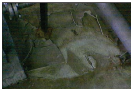
Delaminated fiberglass mat polyester.
