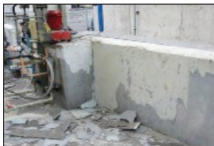
Failed coating after spills.
