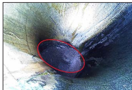
Dark scale formation on unlined section.
