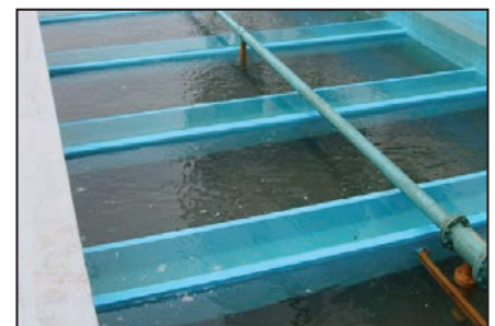
Sand filter in service.
