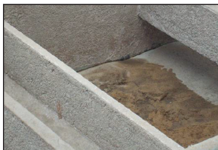
Drained sand filter vessel.
