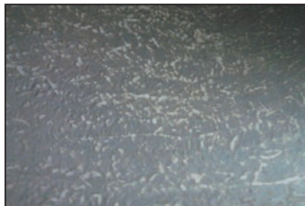
Corroded tank internal surface.
