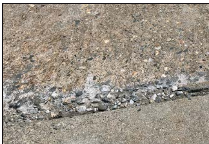
Damaged concrete surface.
